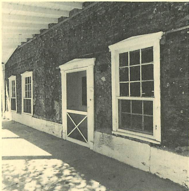
Front facade of the Tully House ready to be replastered. Hope Curtis
