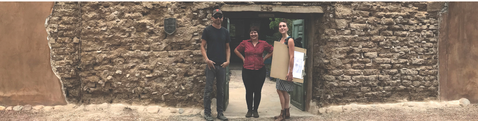
El Zaguán entryway and front wall repairs with 2018 intern Jay Dickason, HSFF Staff Mara Saxer and HSFF Researcher Kelly Davis, September 2018
