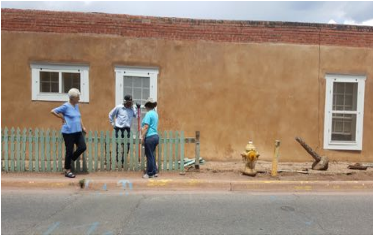
HSFF Staff Jacqueline Hill and Bobby Wilson and preservation intern Janell Keyser inspect the fence outside El Zaguán before beginning repairs
