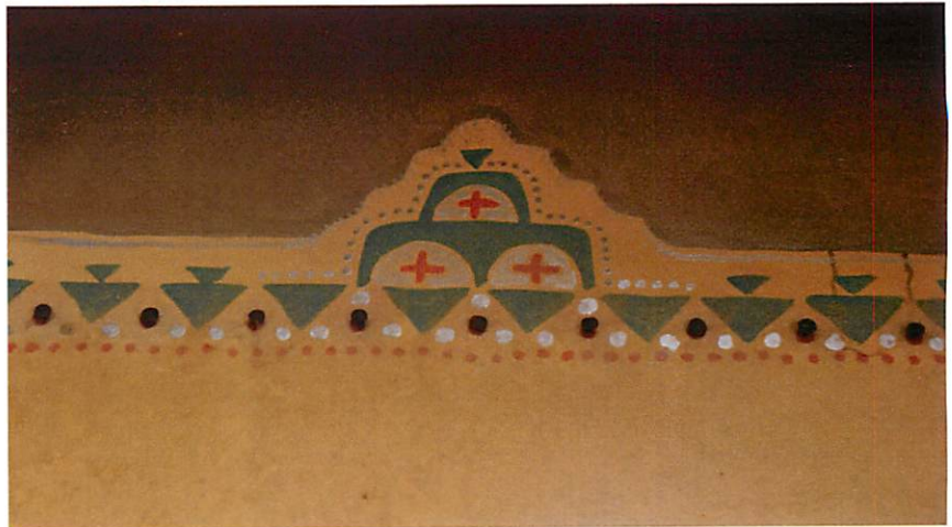
Frieze detail in the octagonal foyer. The line of dark circles are nail heads from which prints and paintings were hung. Therefore, no additional penetrations were made in the decorative finish below. Photo by Hope Curtis.
