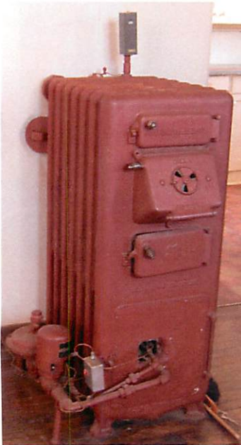
The original 1923 Arcola boiler manufactured by the American Radiator Company was still operating in 2009. Originally coal fired, it was converted to gas in the 1930s. During the restoration, a new boiler was installed in the basement below and the old Arcola now functions as a "radiator".
